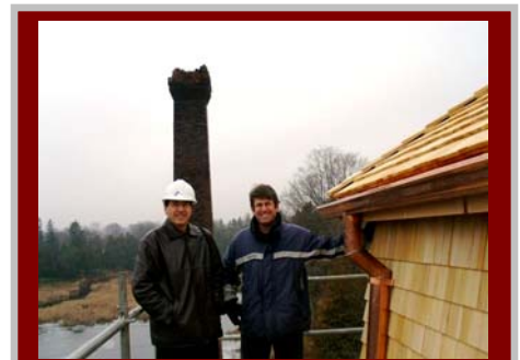
Jordan and Jeremy Grant beside the newly-restored tower roof at Alton Mill
